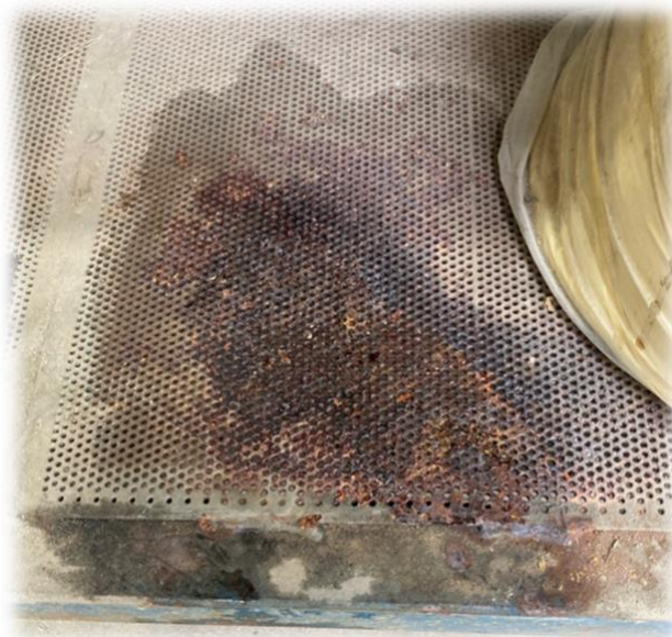
Fig. 8: Corrosion of metal surface at Corowa feed mill after long term storage of calcium nitrate product.
