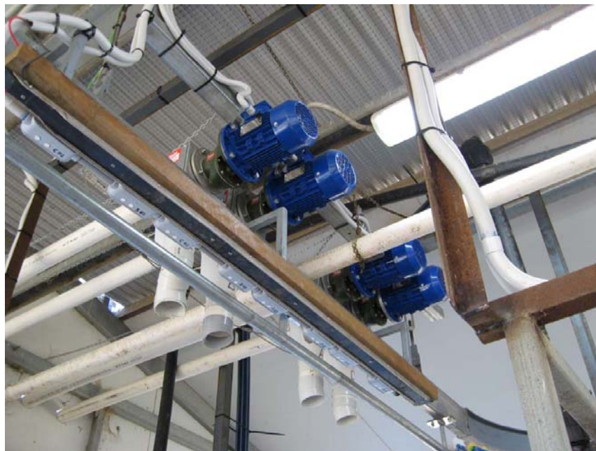
Figure 3. Loading station for the FDU showing the four delivery augers.
