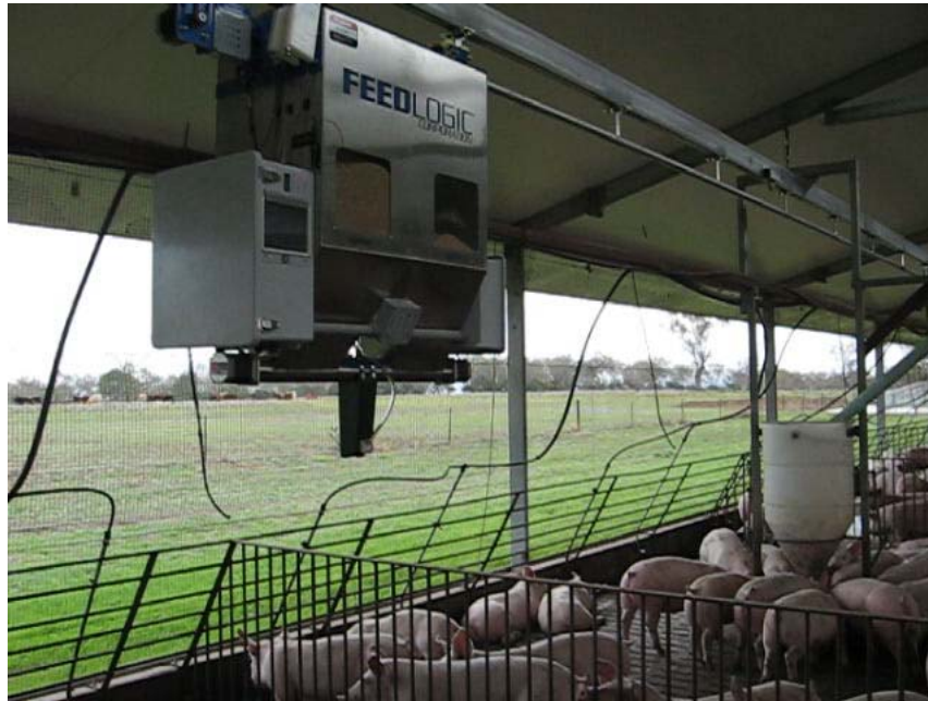
Figure 2. FEEDLOGIC FDU showing running rail.
